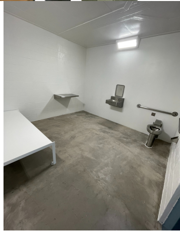
ONE OF 60 CELLS WITH ADA COMPLIANT SINKS, TOILETS AND GRAB BARS FOR WHEELCHAIR USERS
